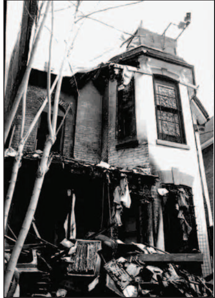
Fig. 1: The Zündel residence in Toronto after the arson attack on May 7, 1995.
